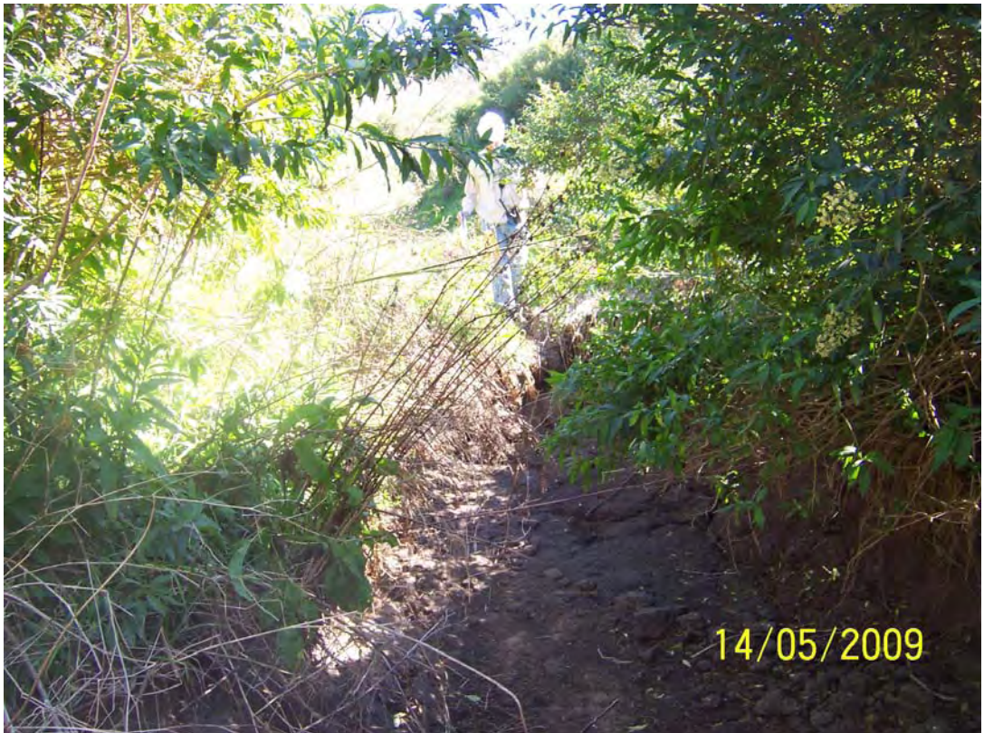
Plate 11: Minor Scour at About Ch.750 Looking Upstream
